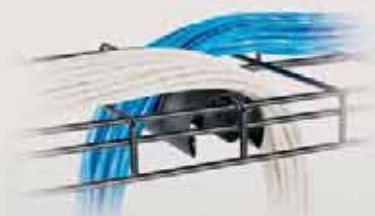
Route redundant ("A" and "B") cabling into adjacent cabinets with a single waterfall.
